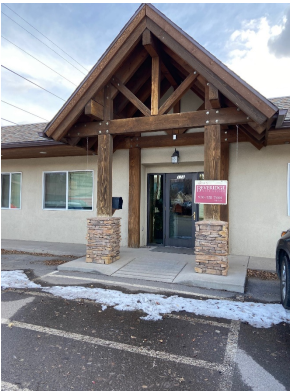
Figure 2 – Front of building – encroaching entry structure
