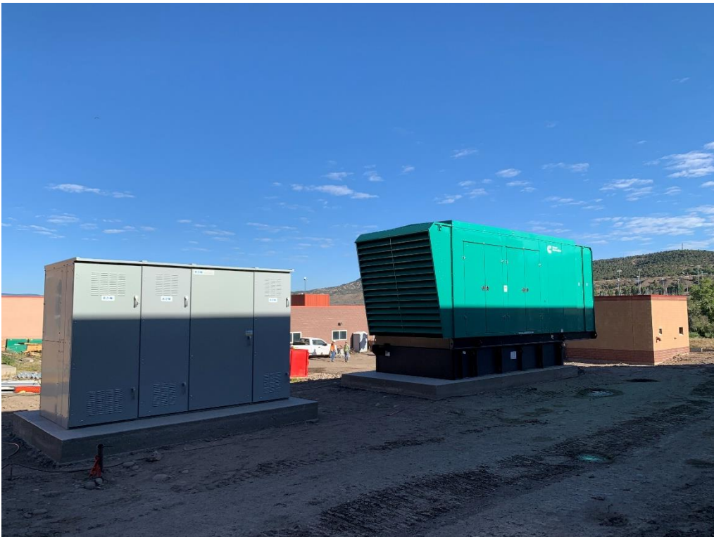
Generator/Transfer Switch Set 07-09-20
