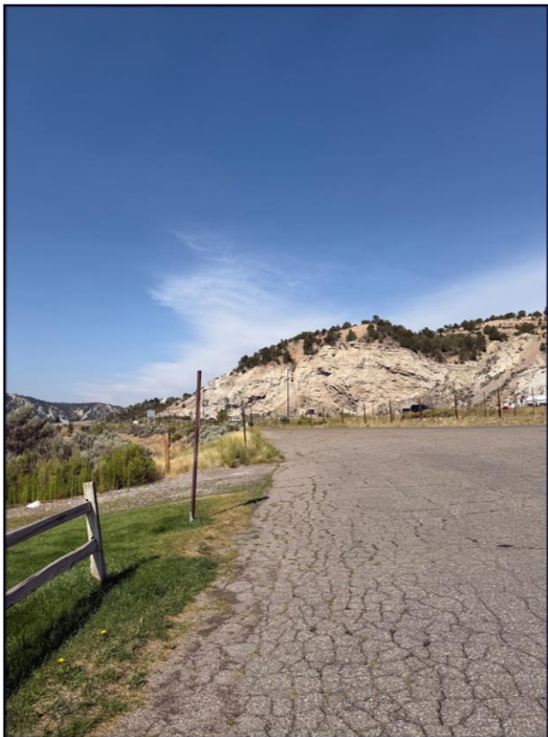
MISSING SIDEWALK TO RIVER PARK
