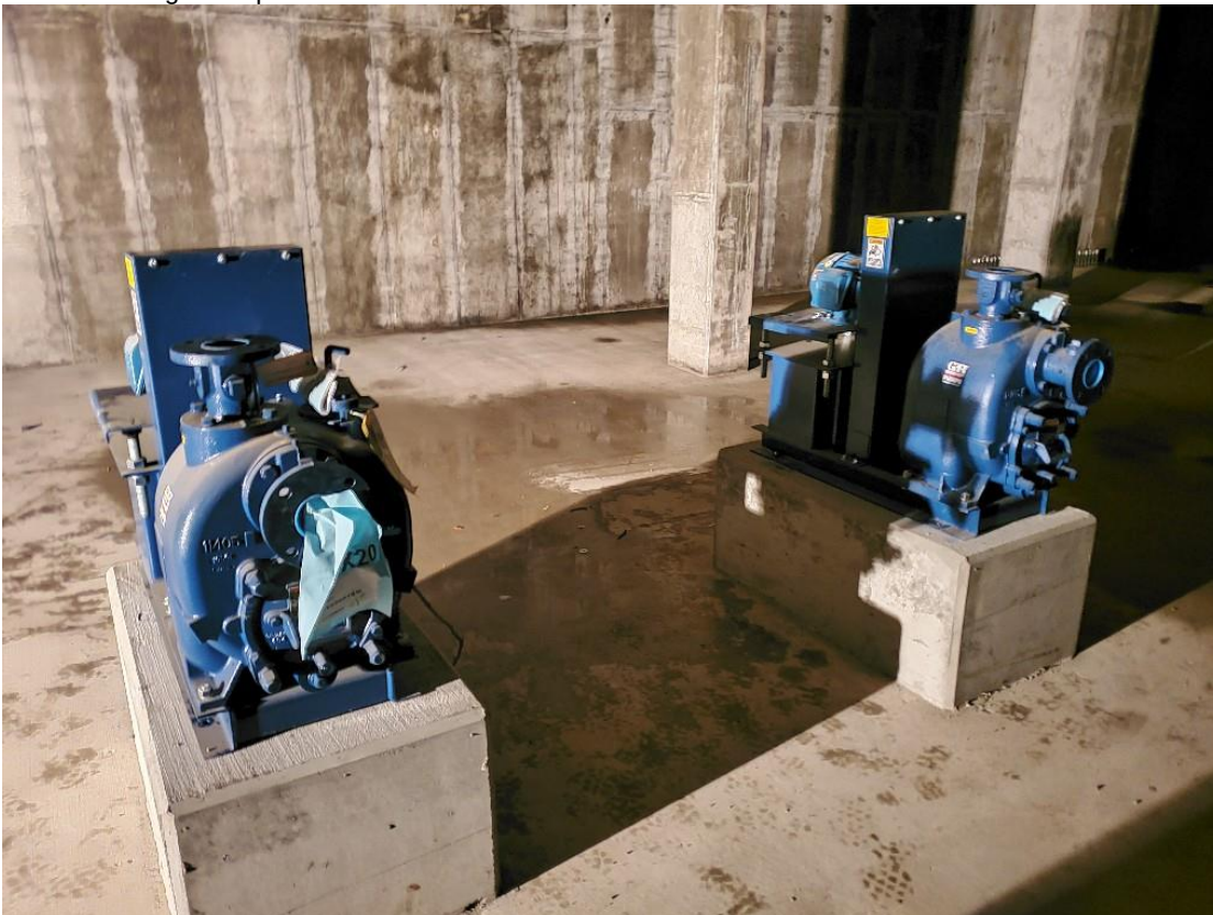
Residual Sludge Pumps 2-05-20
