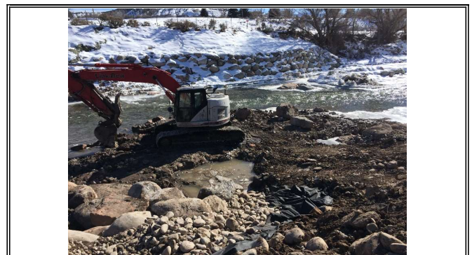
Eagle County Irrigation Intake and Maintenance Ramp
