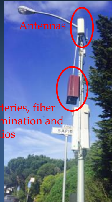
Light Pole – No Ground Cabinet
