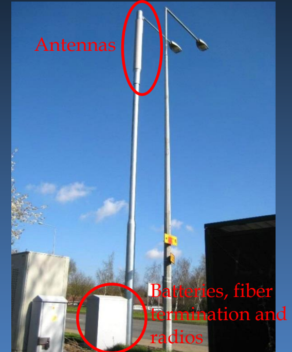
Light Pole – Ground Cabinet
