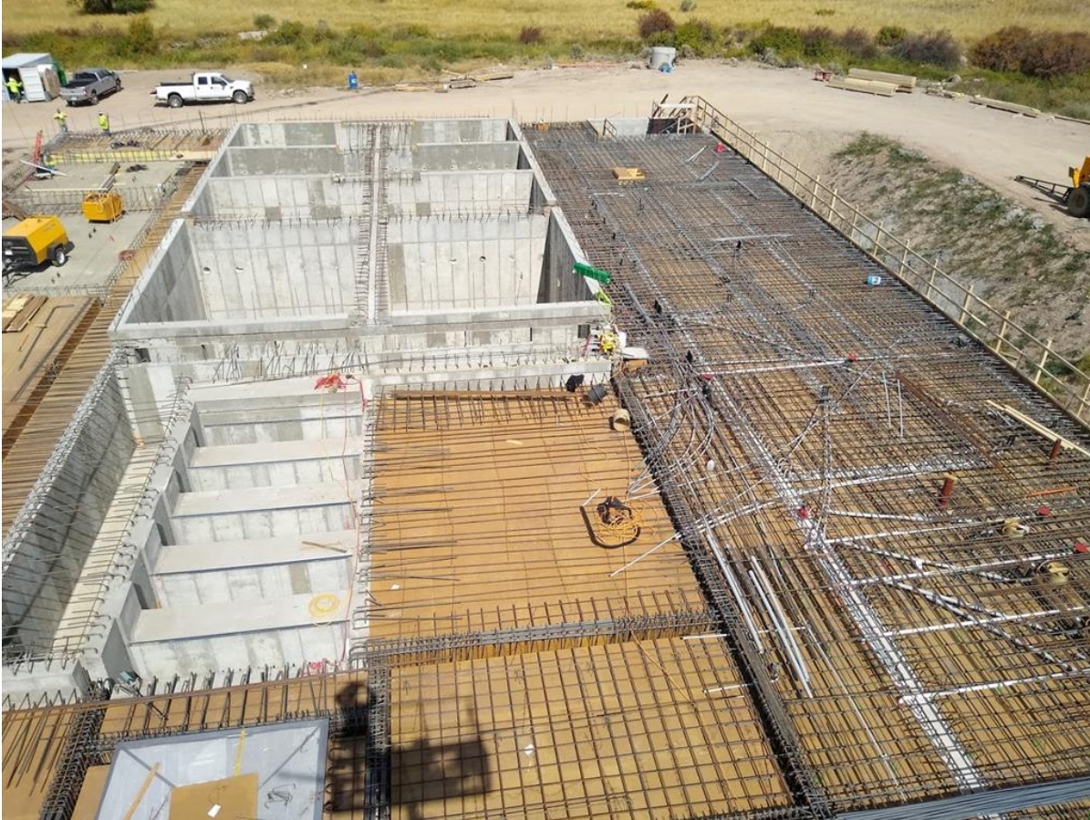
Water Treatment Building Deck 10/1
